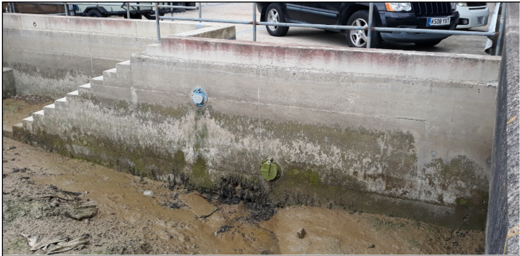
Flood gate to basement car park
